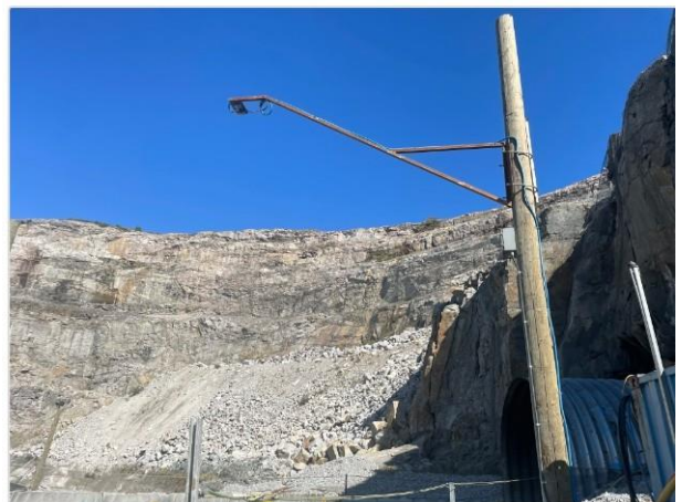
Surface scanner installation - North Portal
